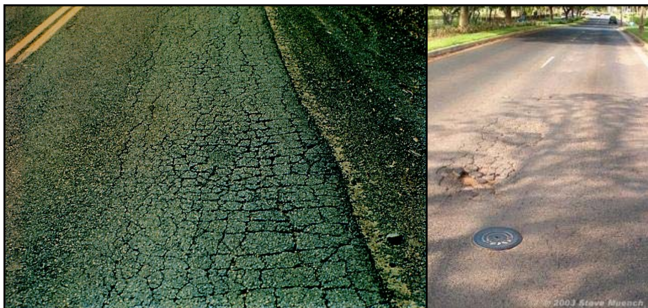
Figure 10: Fatigue cracking (left). Pothole caused by fatigue cracking (right) [20]
