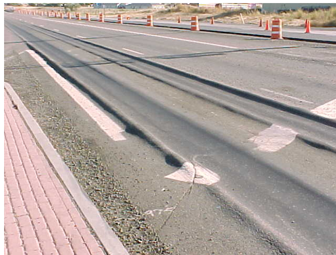
Figure 9: Severe rutting in flexible pavement [19]
