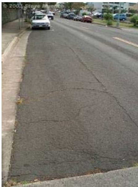
Figure 11: Block cracking, type of thermal cracking [21]
